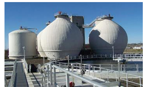
Level measurement with laser in digesters.
