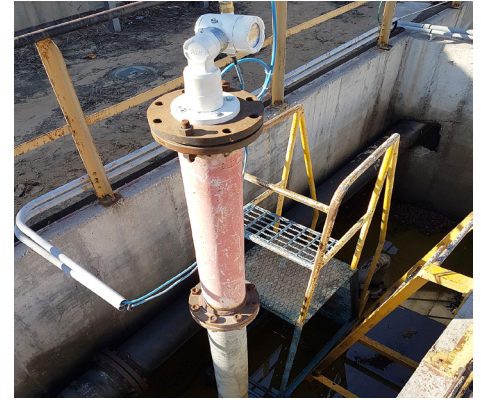
Oil tank level measurement through a long narrow pipe with laser.
