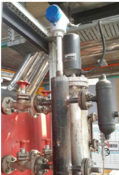
OPTIFLEX 8200C used for level measurement of softened water in industrial boilers.
