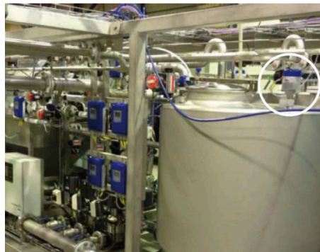
OPTIFLEX 1100 C used at a water purification system skid.
